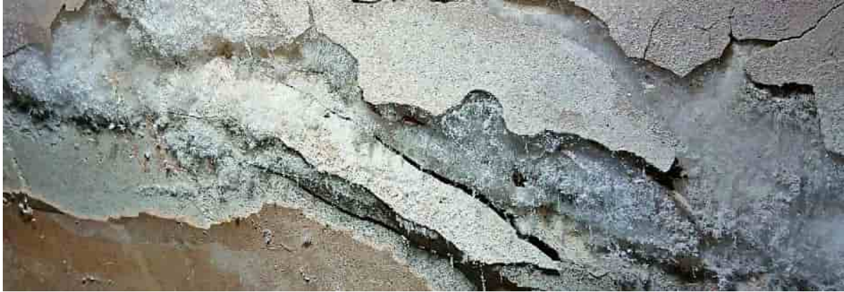
Crystallizing salts breaking down the plaster
