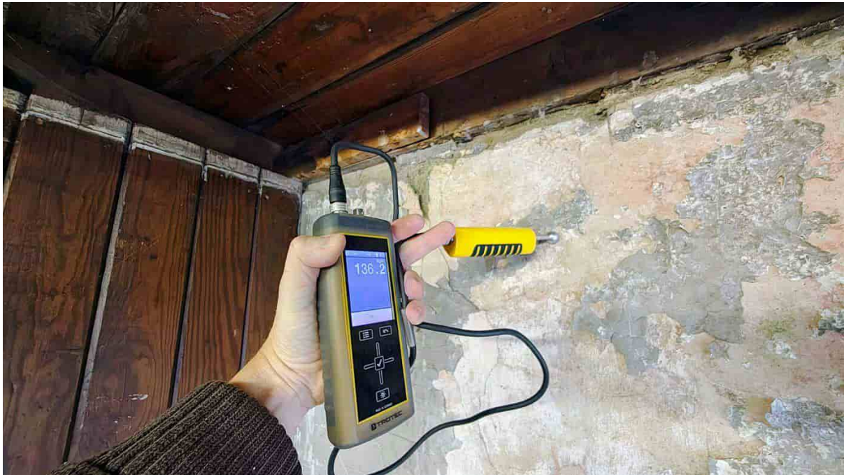
West Wall – plaster high elevation, high reading: 136
