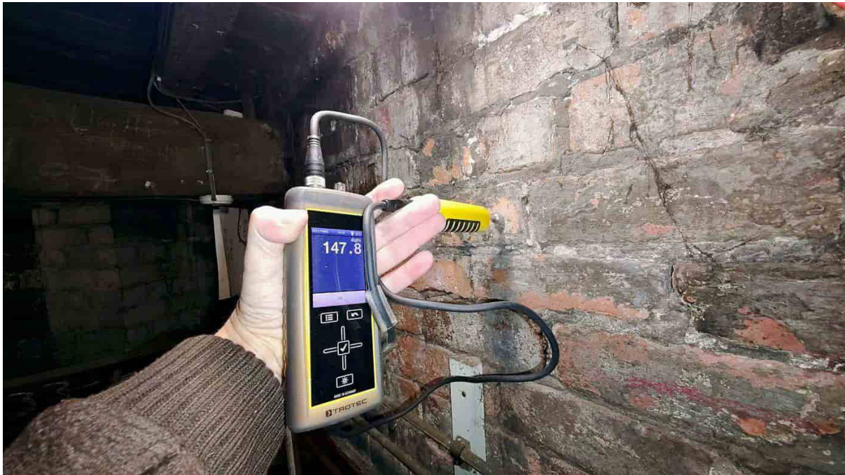
West Wall – external, high reading: 147
