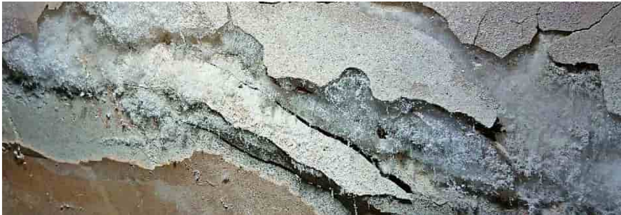
Crystallizing salts breaking down the plaster
